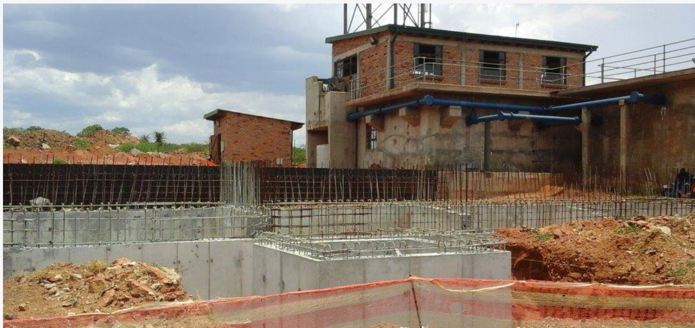
Molepo Water Treatment Works: Polokwane Local Municipality
