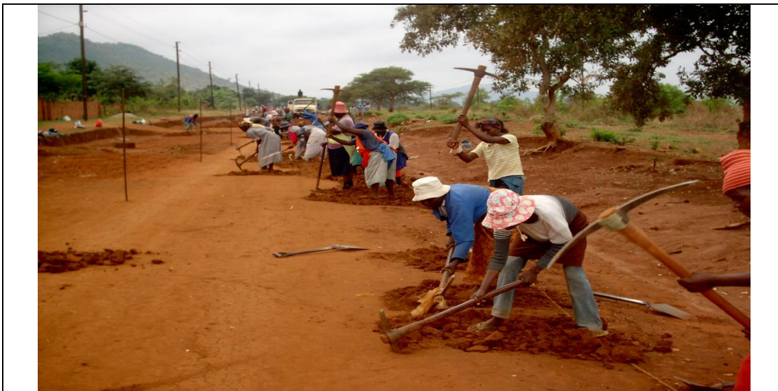
Picture 5: Labour intensive methods create jobs and ensure skills transfer to communities
