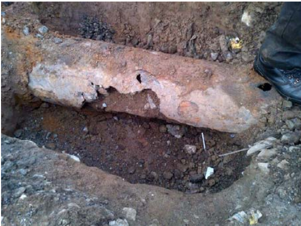
Above: Cambridge Street pipe crossing sinkhole
