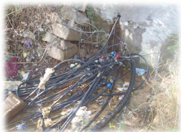
Unauthorised water connections
