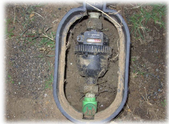
Domestic metered connection
