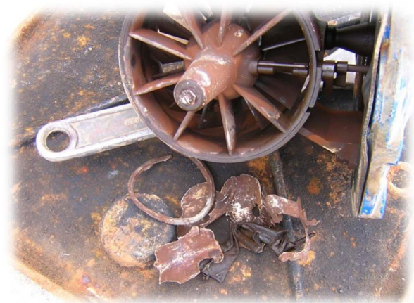
Debris caught in the meter mechanism will cause meter error
