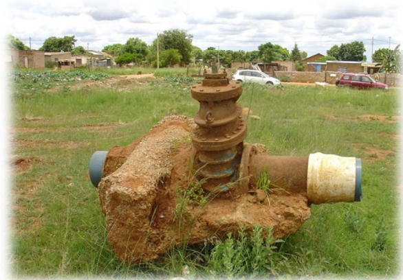
Isolating valve which had to be replaced after continuous opening and closing
