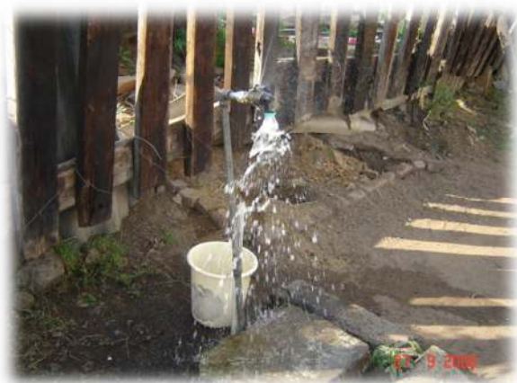
Leakage from an uncontrolled public standpipe
